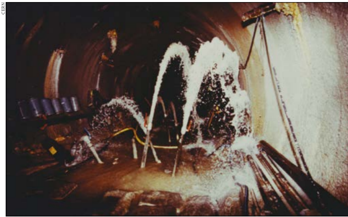
Fig. 1. Blasting the LEP tunnel under the Jura mountains caused water to burst into the tunnel, forming an underground river that took six months to eliminate.
